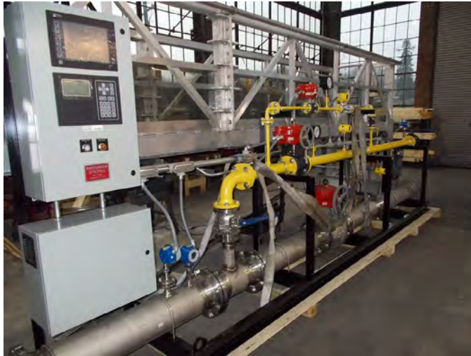
Natural Gas and Digester Gas Blending Station with Preferred PWC controller and 10" Color Touchscreen
