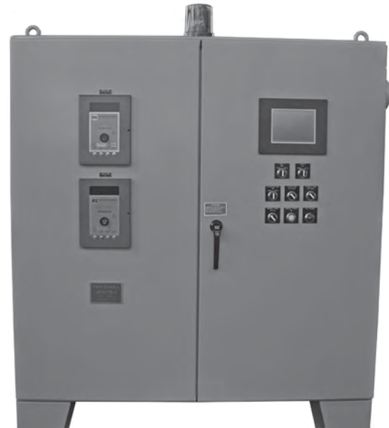
Custom Fuel Delivery System
