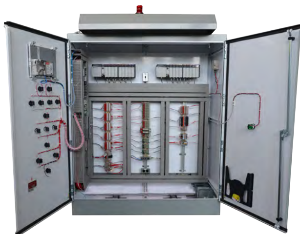
PLC-based flame safeguard and combustion controls system in a free-standing enclosure
