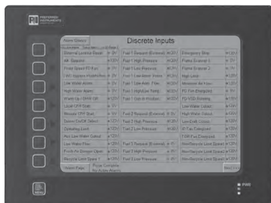
Controller I/O screens help troubleshoot problems
