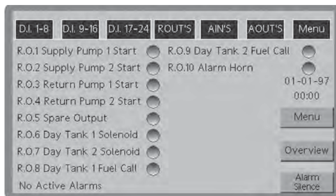
Typical relay output screen helps troubleshoot controlled devices.
